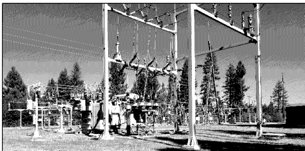
Figure 30. North Truckee Substation
