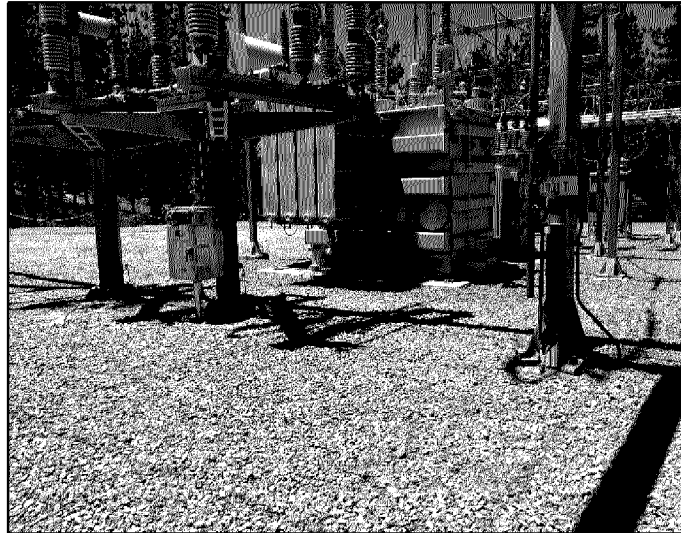
Figure 27. Round Hill Substation
